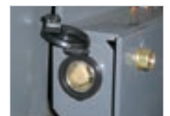
Backup Power Supply
